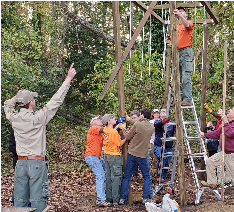
Thomas, '23, leads troops in the construction of a new sensory trail at Maryland Therapeutic Riding.
